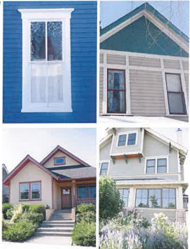
Trim. [1] All windows and doors should have side trim and head casings [2] Trim should be at a minimum 3½ inches wide and project no less than a ½ an inch from the wall.
