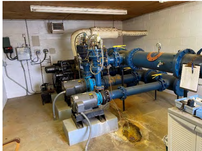
Figure 4-20 | Polk Pump Station
