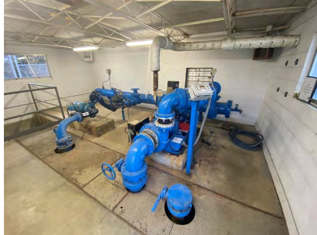
Figure 4-22 | Monmouth Street Pump Station
