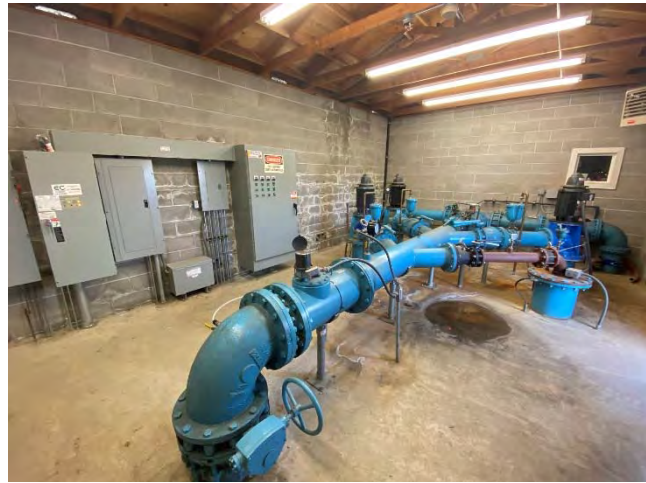
Figure 4-21 | South Pump Station
