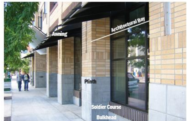
Large storefront windows, awnings, and a tall ground floor height enhance the character of the ground floor. Plinths, a projected soldier course, and the bulkhead articulate the base.
